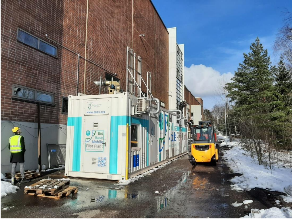
Figure 5 BBMPP unit with exhaust pipes on the roof installed in March 2023.
