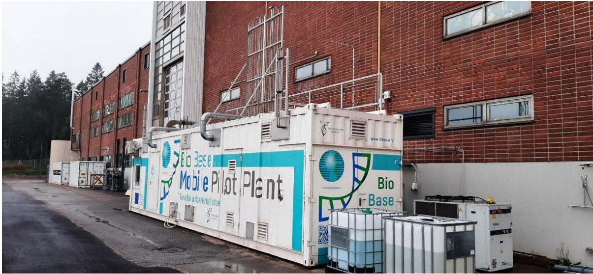
Figure 6 Mobile gas fermentation unit fully operational during May 2023.
