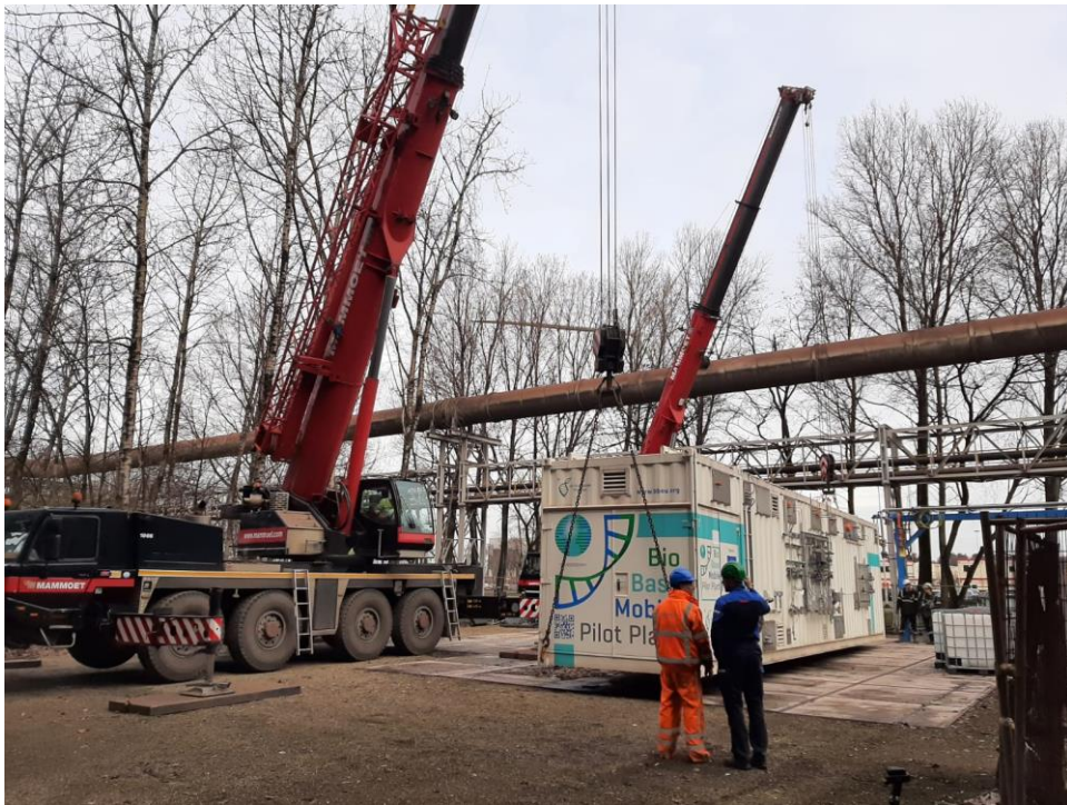
Figure 1 Lifting in place of the BBMPP at the site of Arcelor Mittal Ghent for its relocation.
