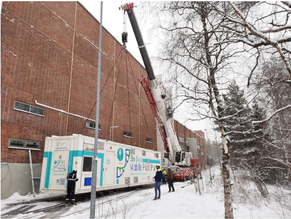
Figure 4 Placement of the BBMPP unit at VTT's Bioruukki site on 27th of March 2023.
