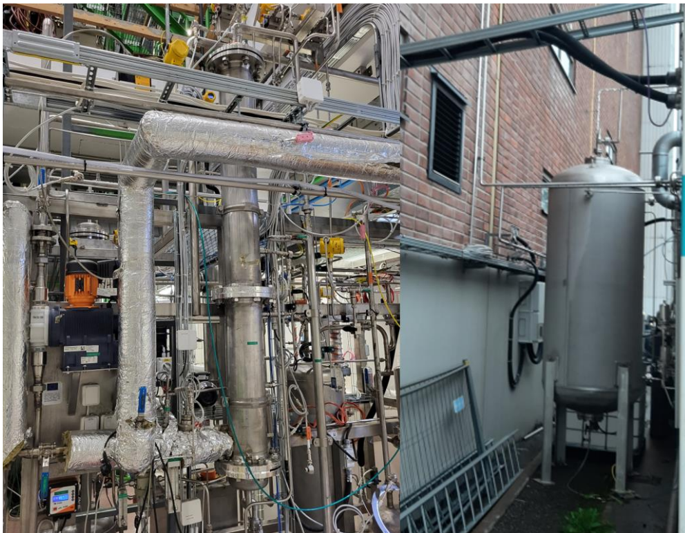
Figure 9 The scrubber that was used in ultra-cleaned, acid-scrubbing and alkaline scrubbing campaigns on the left side. The cleaned syngas was fed to the buffer tank shown on the right side.
